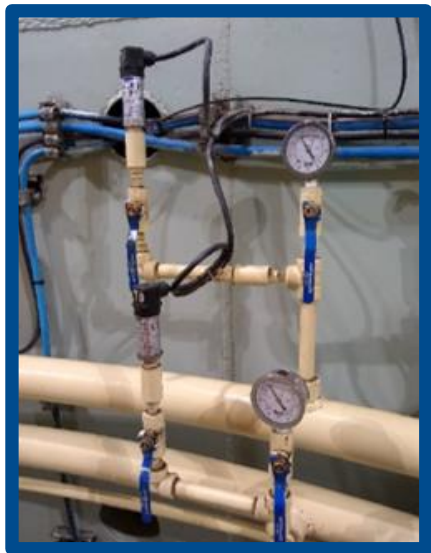
Measurement of opening and closing pressures of WG servomotors
